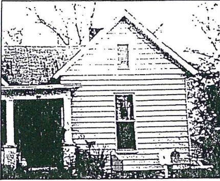
Synthetic siding which has disguised significant architectural features.
