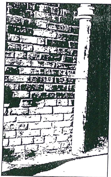
Masonry suffering from water damage.
